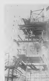
The Marine observation tower gets a boost upward as construction begins on a higher tower. In the center is the old control office. Around, and through it, is being placed the structure for the new 75 foot tower.
